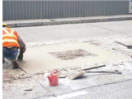
KFDN-SES800 應用在香港道路緊急修補工程上 Used for emergency road repair in Hong Kong
